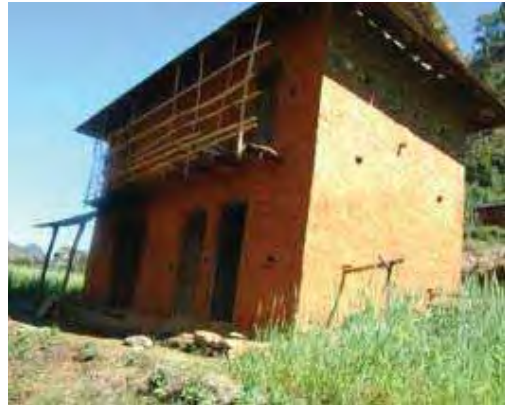
Affected House at Ch 0+750 (Mijhing VDC)
