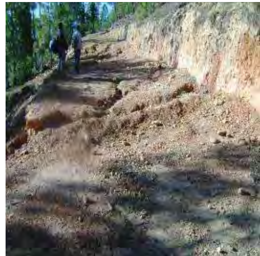
Soil erosion (Ch. 5+400)
