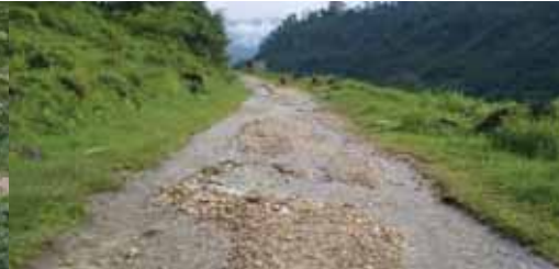
Need Better water management At chainage 0+570
