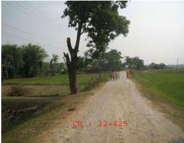
Affected Peepal tree at Ch 22+425
