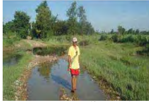
Water Logging at Road(Ch-15+730)
