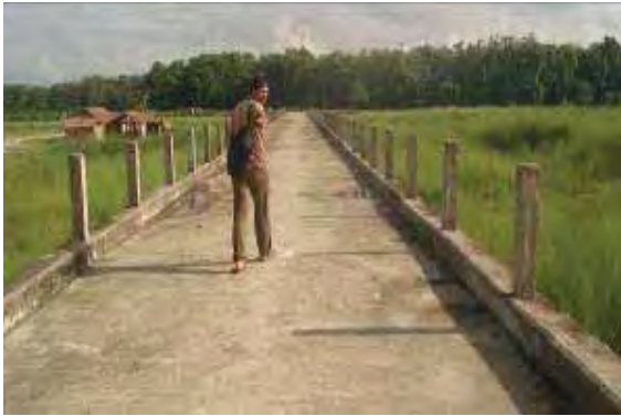
Starting point (End of this damaged bridge)
