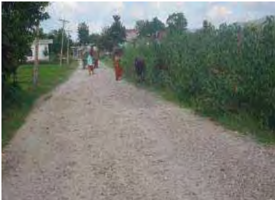
Present road Condition (Ch. 2+100)
