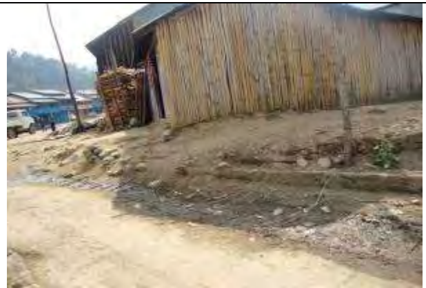
PHOTO NO. 10 Affected house at Ch (26+000 to 26+010)
