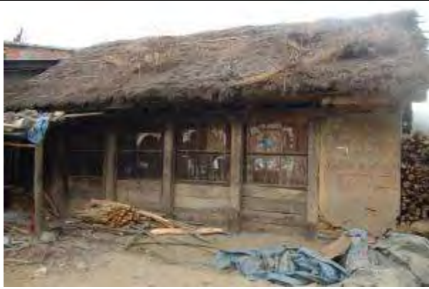
PHOTO NO. 7 Affected house at Ch (0+220 to 0+227)
