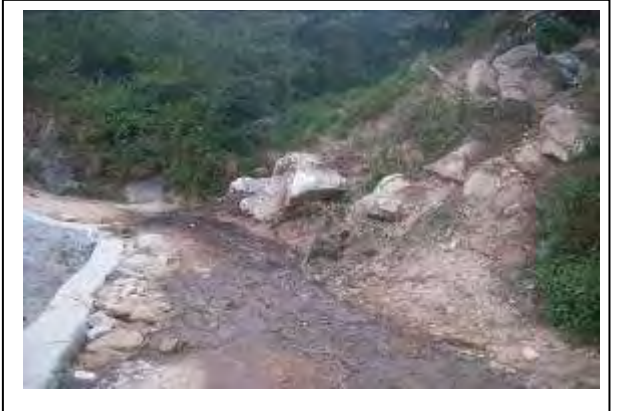
PHOTO NO. 12 Kali gairi, Rati Khola, Budhabare-9 need to be widen by clearance of debris and to stabilize the landslide.
