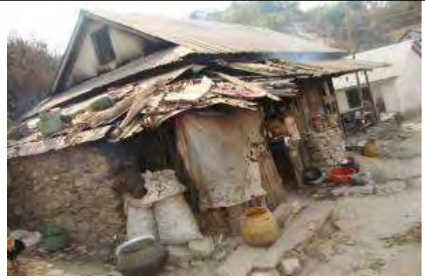
PHOTO NO. 8 Affected house at Ch (5+040 to 5+051)
