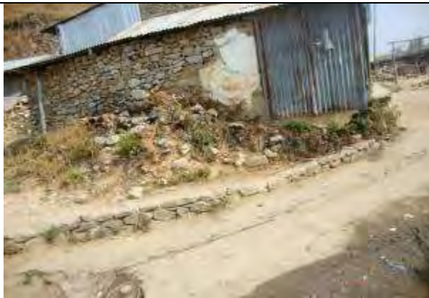
PHOTO NO. 9 Affected house at Ch (26+000 to 26+010)
