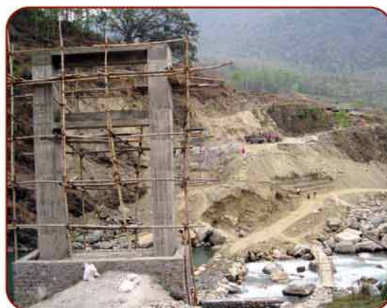
Right Bank view of Motorable Suspension Bridge underconstruction over Modi River on Dobilla- Phalebas Rural Road at Parbat District
