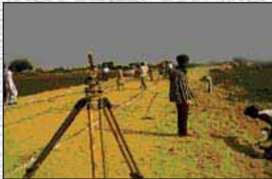
Preparation for construction of granular Sub-base: Dabra Jangipur Road to Gadi, Length 4.00 Km. Cost 63.89 Lakhs. District Gwalior, Madhya Pradesh.
