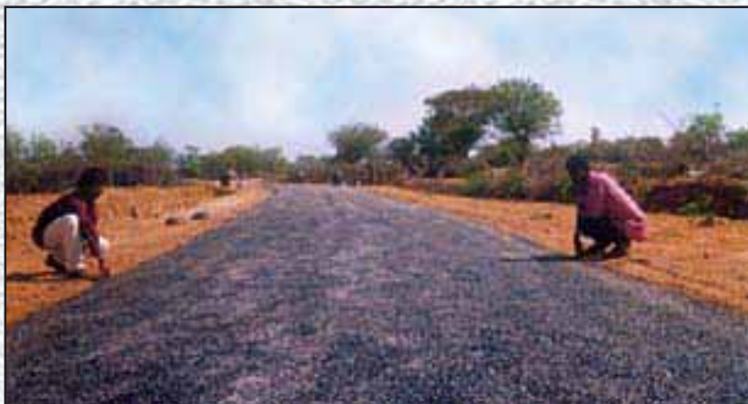
Premix carpet after compaction: Alampadi to Ivanur Road, Length 5.20 Km., Cost: 53.36 Lakhs, District Cuddalore, Tamil Nadu.
