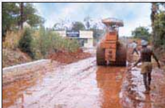
Wet rolling of Water Bound Macadam Road after screening and binding material has been spread: B.C.C. Road to Sengalipallam, District Karur, Tamil Nadu.
