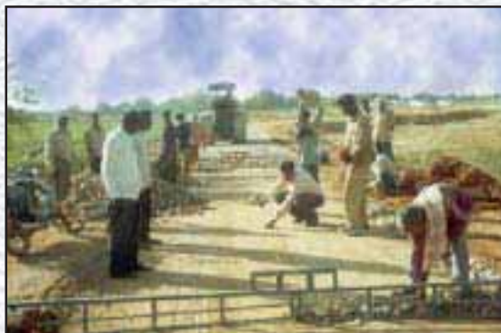
Laying of metal with the help of Camber Board: Length: 4.20 Km. Cost 64.56 Lakhs. District Gwalior, Madhya Pradesh.
