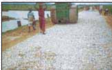
Dry compaction of metal and application of screening material: Narbari Road, Assam.
