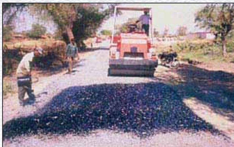
Application of binder after first coat of Surface Dressing: Pimpri Road, Orissa.
