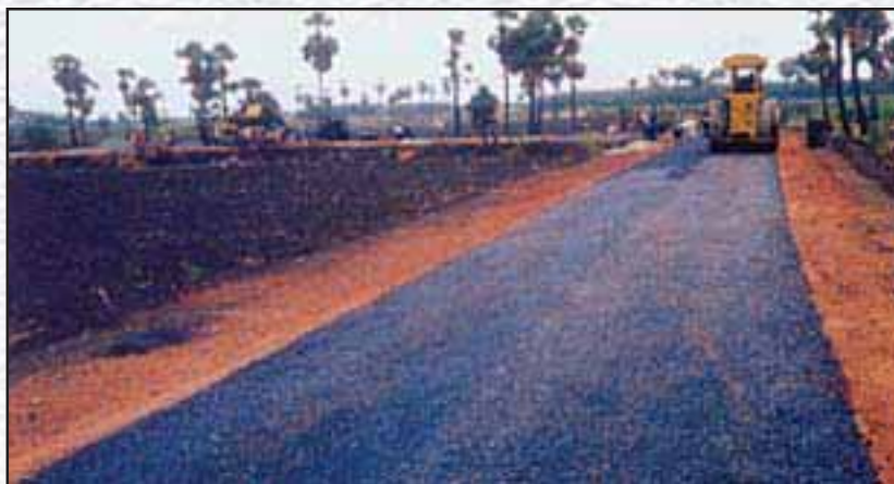
Laying and compaction of 20 mm thick Pre Mix Carpet: Periyavadugapatti to Mangasolipalyam Road, Length 3 Km., Cost: 33.54 Lakhs, District Karur, Tamil Nadu.
